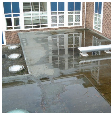
Ponding caused by poor design and maintenance
