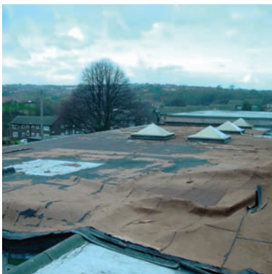
Wind damage resulting from poor design
